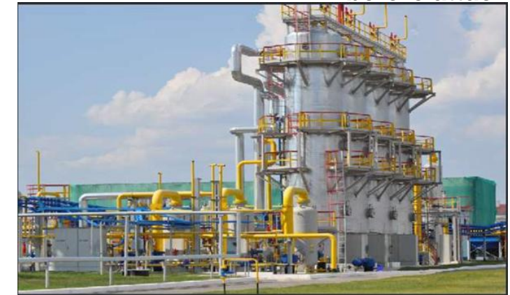
Gas booster compression station before attack
